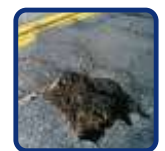
POTHOLES/ DAMAGED PAVEMENT
